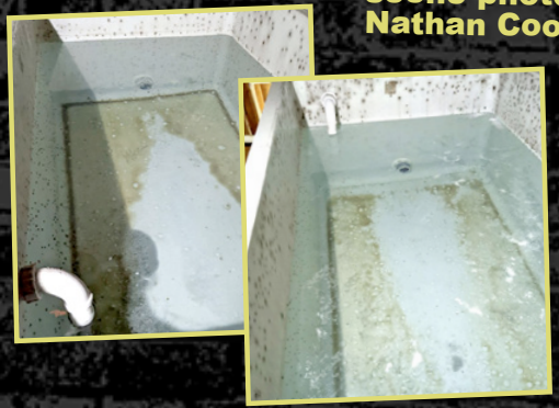
9. Lovely pictures! Thanks to Simon Ostick. Internal of 2 tanks at a leading hotel chain, they had not been completing any inspections! Hope their visitors survived their stay!
