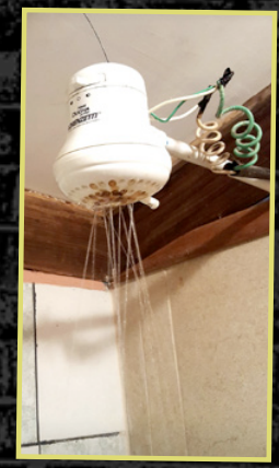
8. This has to be a favourite so far... Sabrina Elliott was lucky to survive her trip to Costa Rica! The showerhead was so covered in bio film, had no water pressure and added to the risk, the instant water heater was built into the head, with live wires! If she touched it, she got electrocuted!
